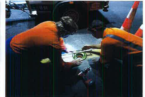
Airways electricians fitting taxiway centerline bases in preparation for taxiway light fitting
