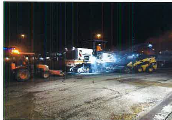
Milling to Taxiway D – note delaminating Base material due to original 1965 construction.
