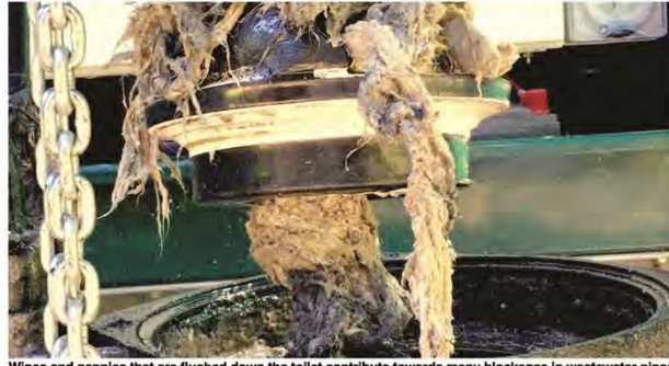
Wipes and nappies that are flushed down the toilet contribute towards many blockages in wastewater pipes.
