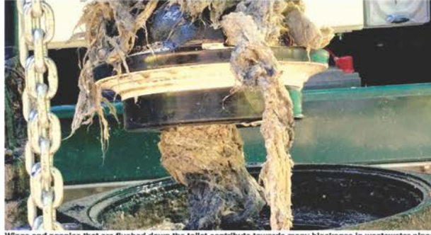
Wipes and nappies that are flushed down the toilet contribute towards many blockages in wastewater pipes.
