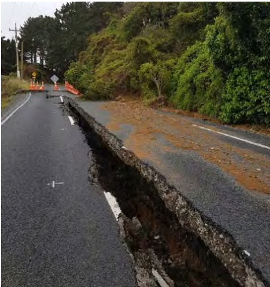
Picture 1: Slump on Koheroa Road, Mercer
