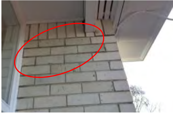
Crack observed in the top corner of the brick veneer adjacent the main entrance
