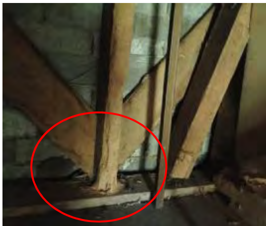
Borer observed in timber supporting the stage
