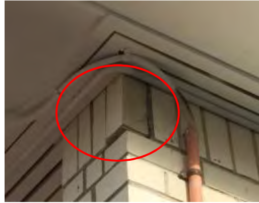
Loose brick observed in the top corner of the brick veneer
