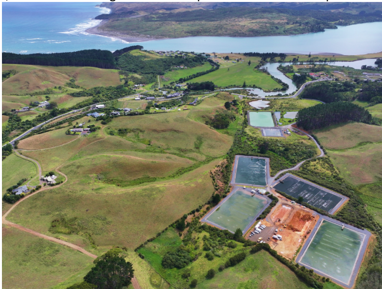
Raglan WWTP MBR Upgrade– Earthworks are underway in preparation for the tank construction. The main activities will be located between the upper ponds.
