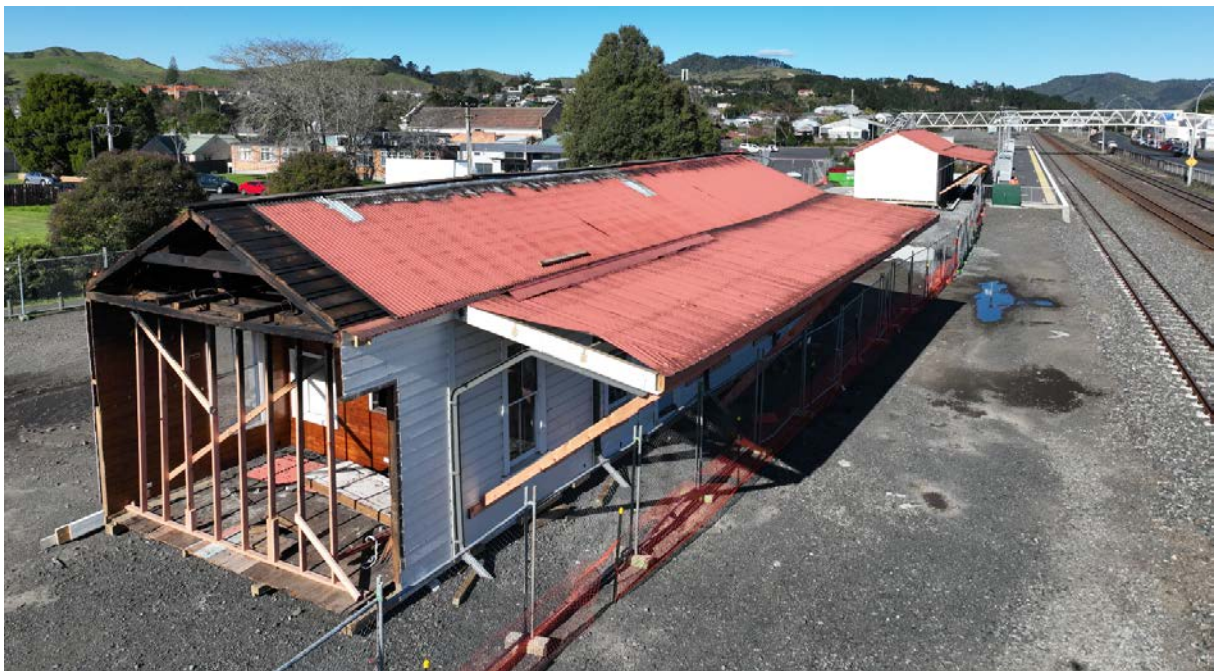
Repairs are now underway on the fire damaged section (photo from June 2023).
