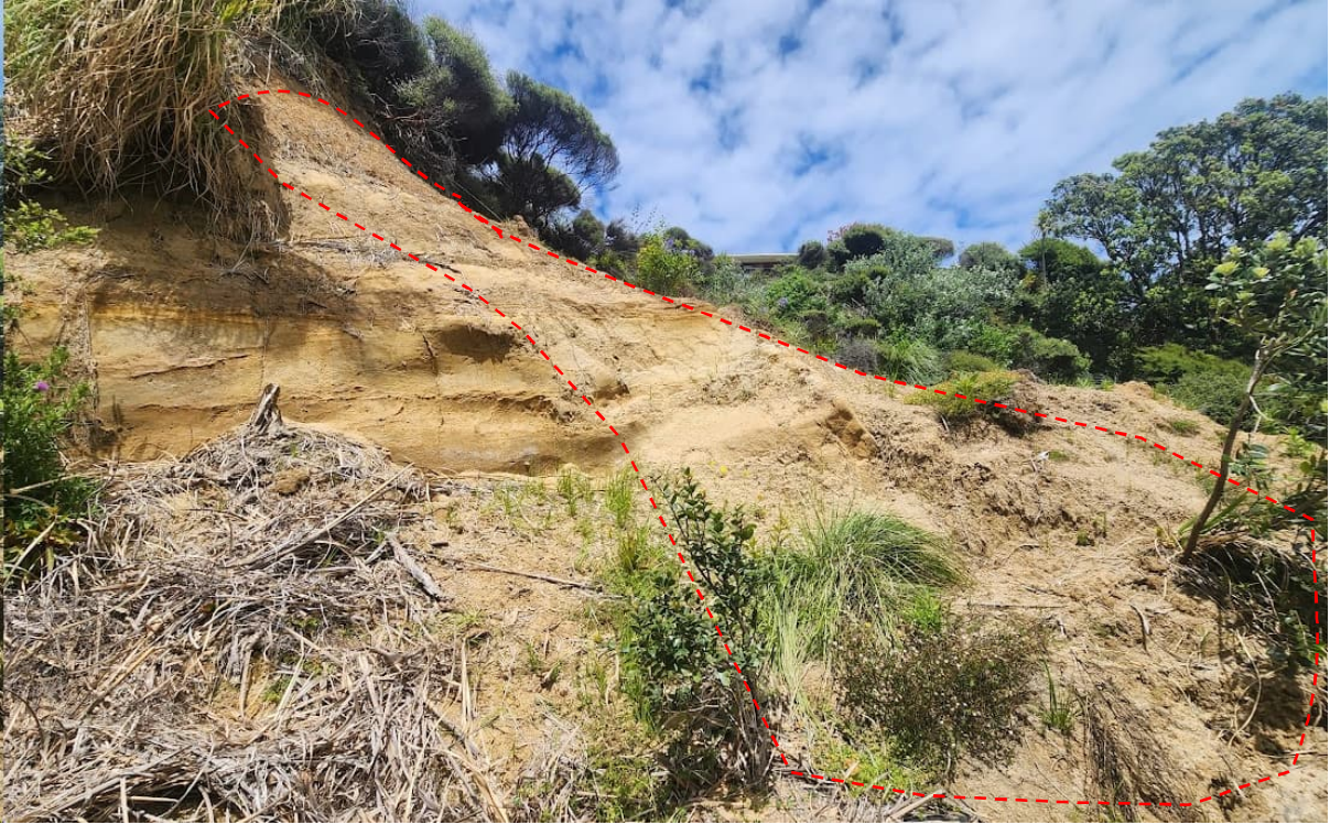
Photograph Appendix B.7: Landslide 2B
