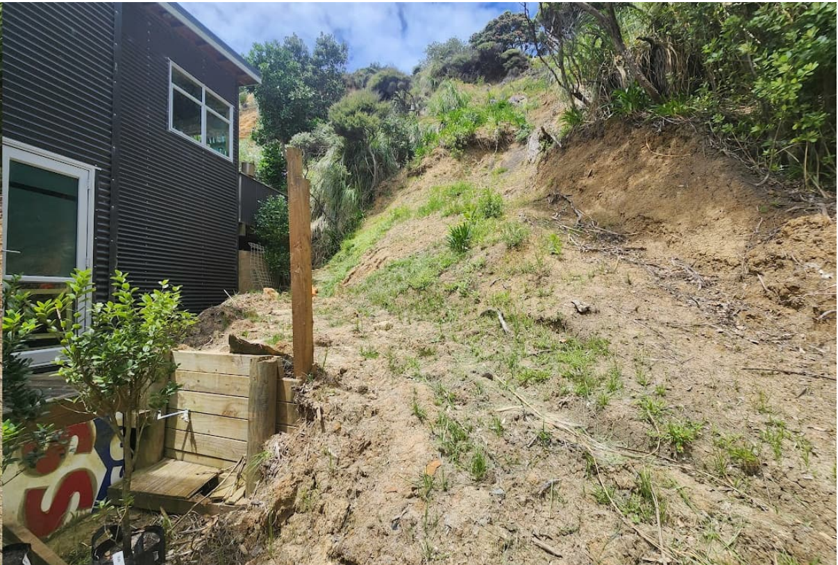
Photograph Appendix B.8: Landslide 2A Inundated land, captured by retaining wall
