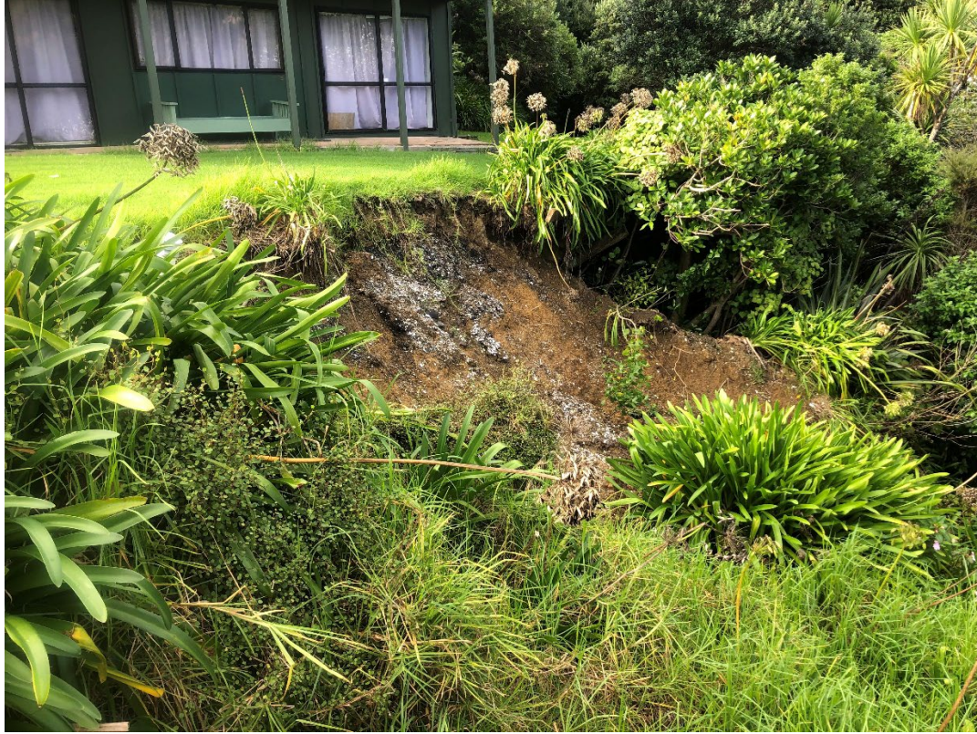
Photograph 11: Landslide 3 below 211 Maunsell Road dwelling
