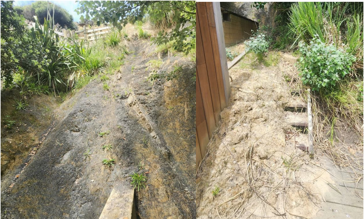
Photograph Appendix B.12: Landslide 1 (left) Murihuku Terrane siltstone (right) Inundated land covering steps
