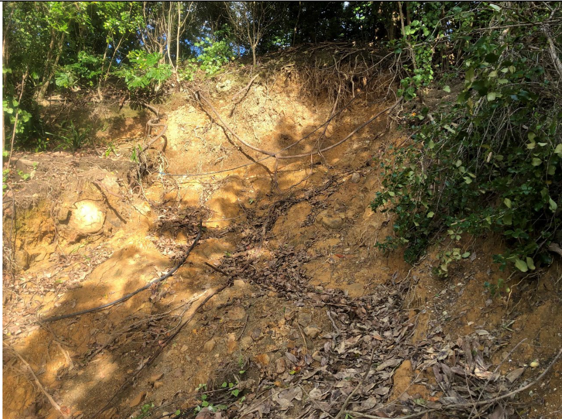
Photograph 2: Landslide within 15 Tuakau Bridge-Port Waikato Road
