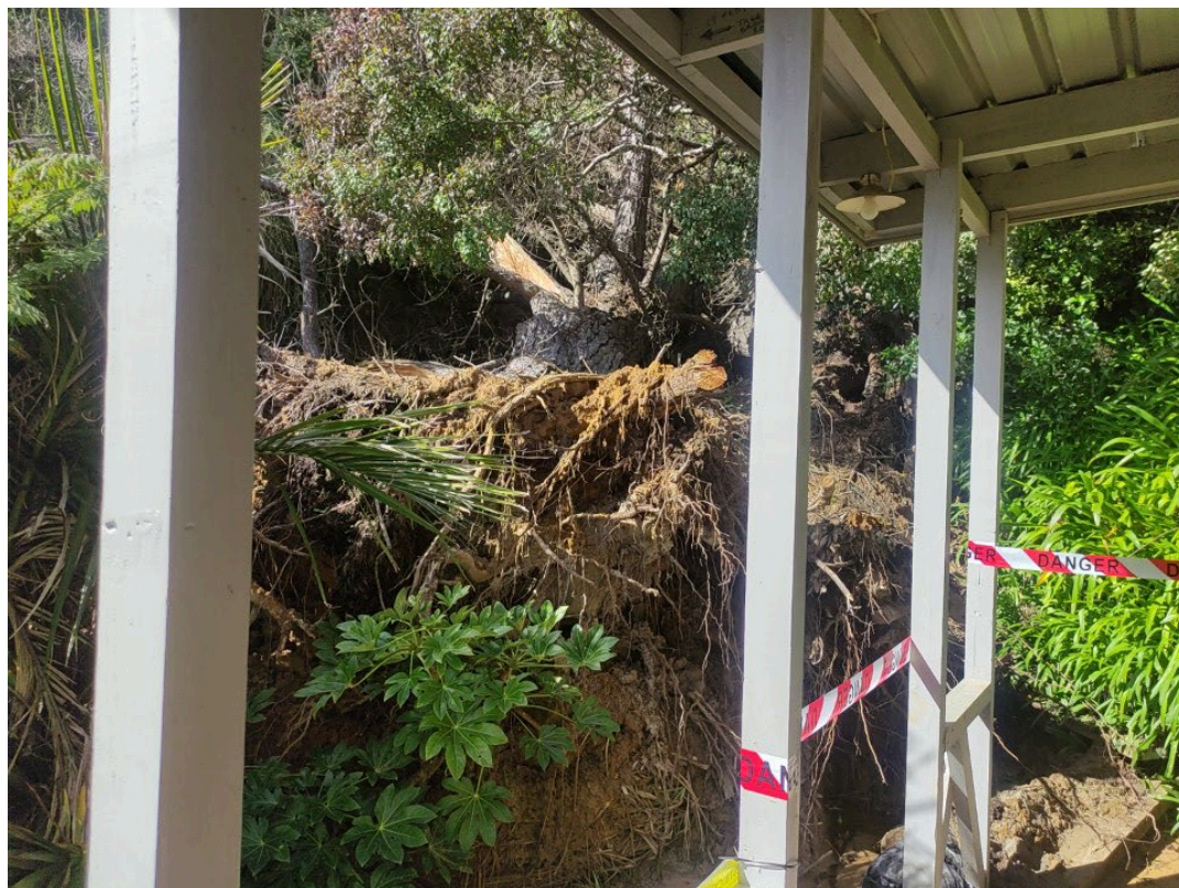
Photograph 14: Debris accumulation adjacent to 201 Maunsell Road
