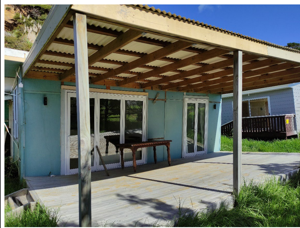
Photograph 15: View of damage to 175 Maunsell Road
