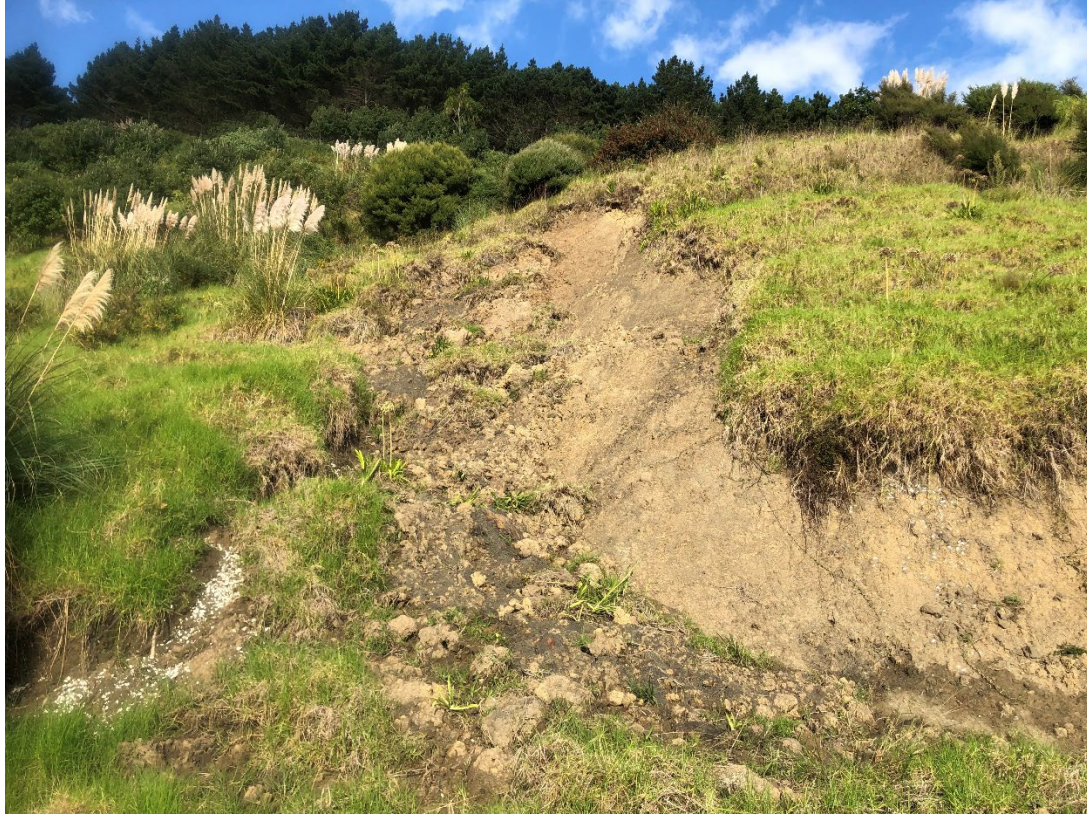
Photograph 9: View of Landslide 13 at the rear of 139A Maunsell Road
