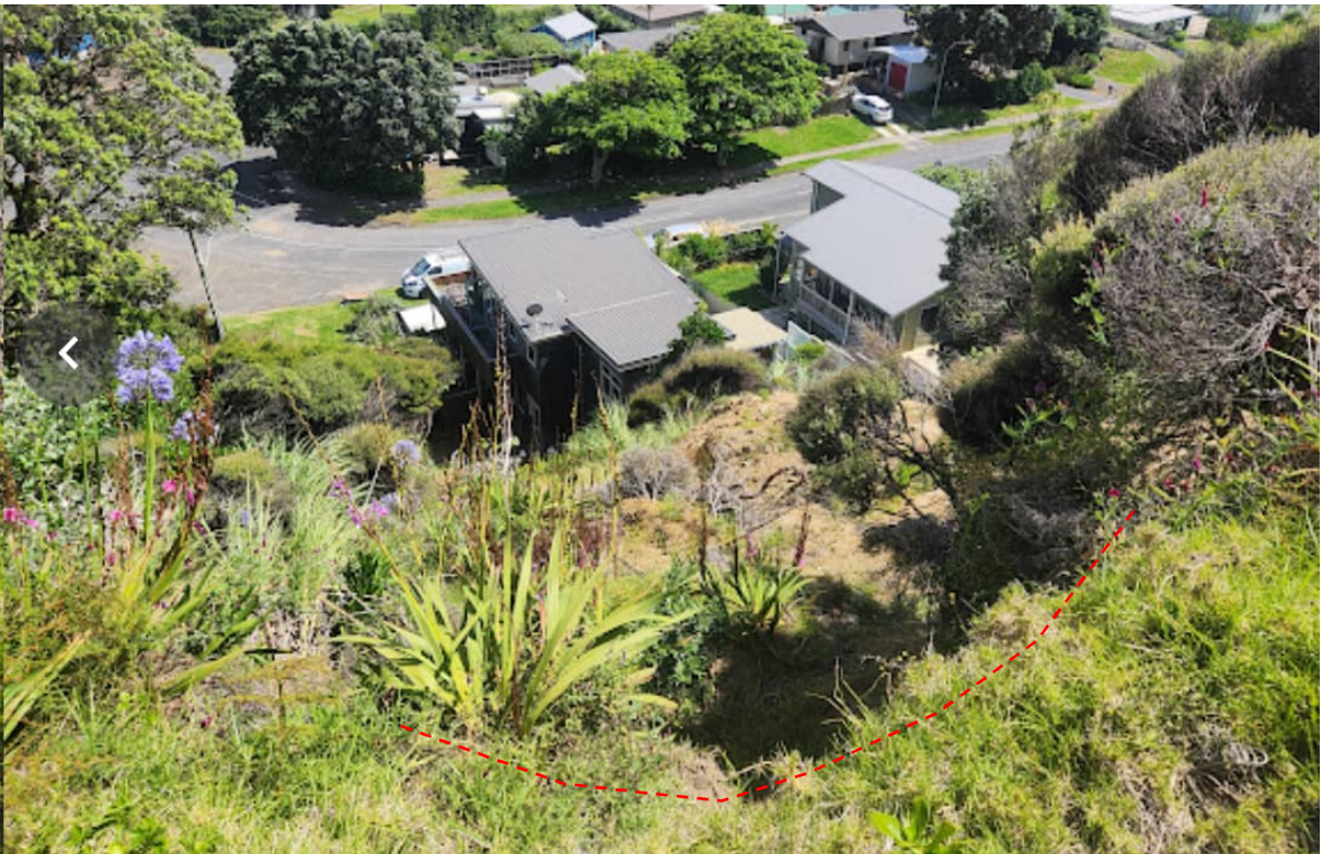
Photograph Appendix B.4: Landslide 2A headscarp
