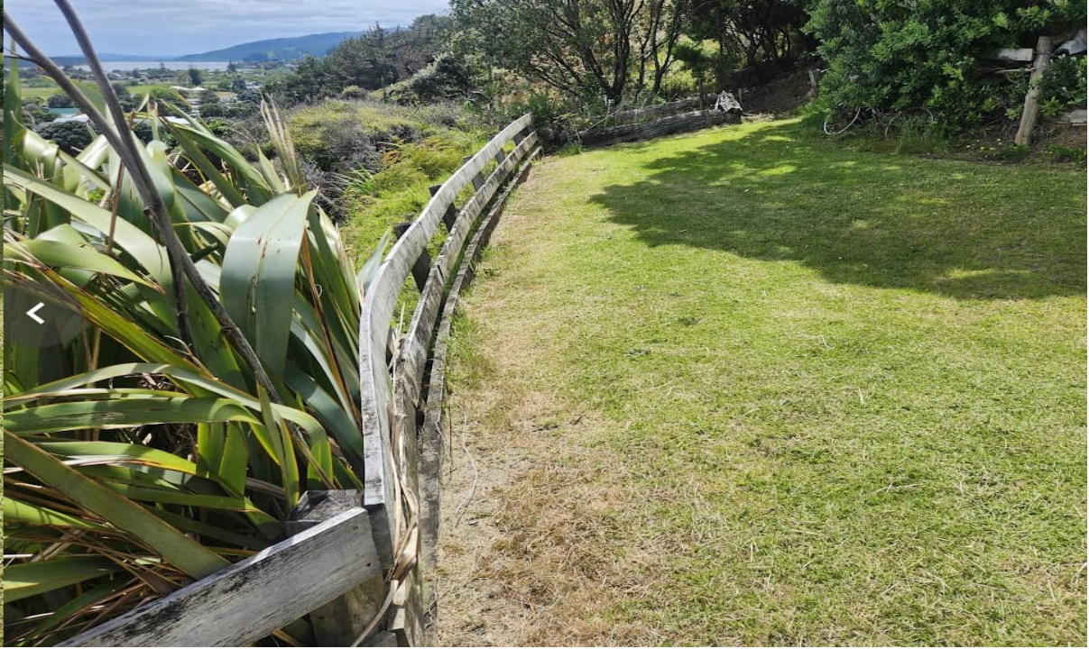
Photograph Appendix B.3: Tilted and bowed fence above Headscarp at 209 Maunsell Road
