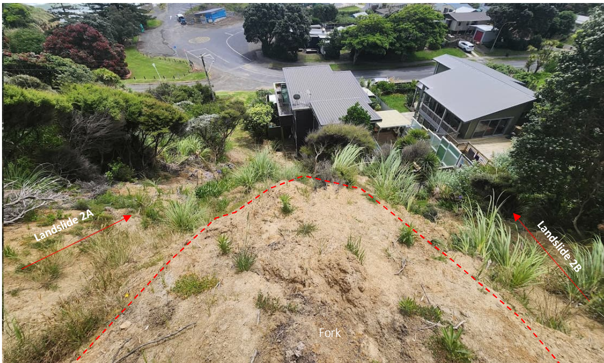
Photograph Appendix B.6: Landslide 2A and 2B
