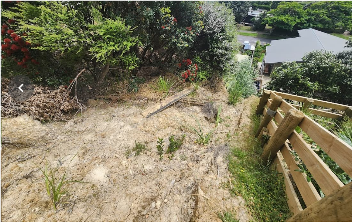
Photograph Appendix B.11: Landslide 1 Excavated land
