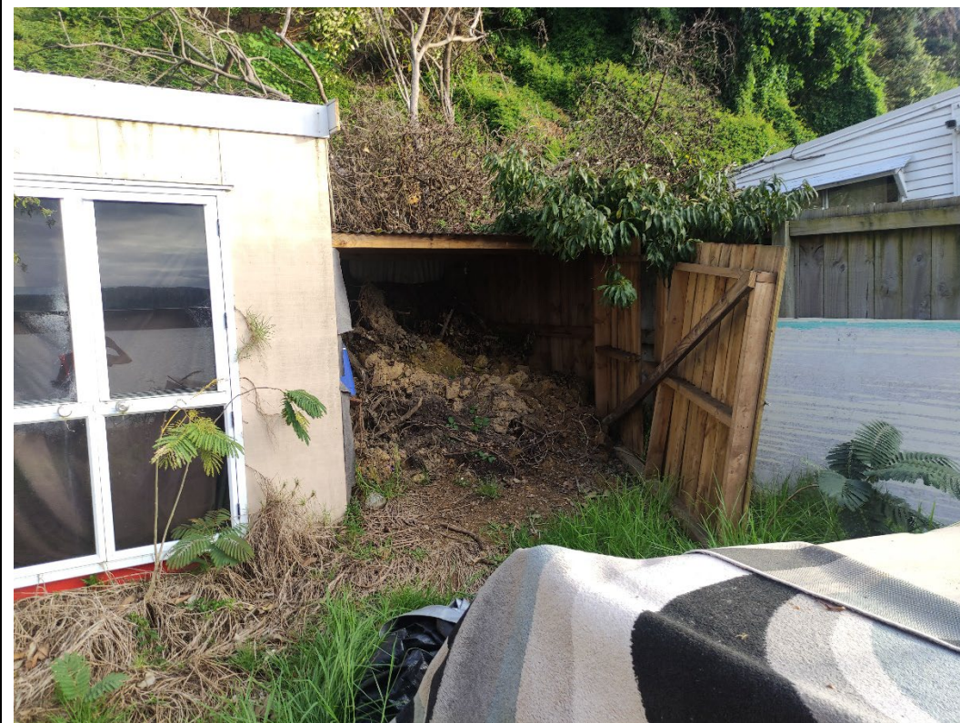
Photograph 8: Damage to shed / car port at 13 Tuakau Bridge – Port Waikato Road
