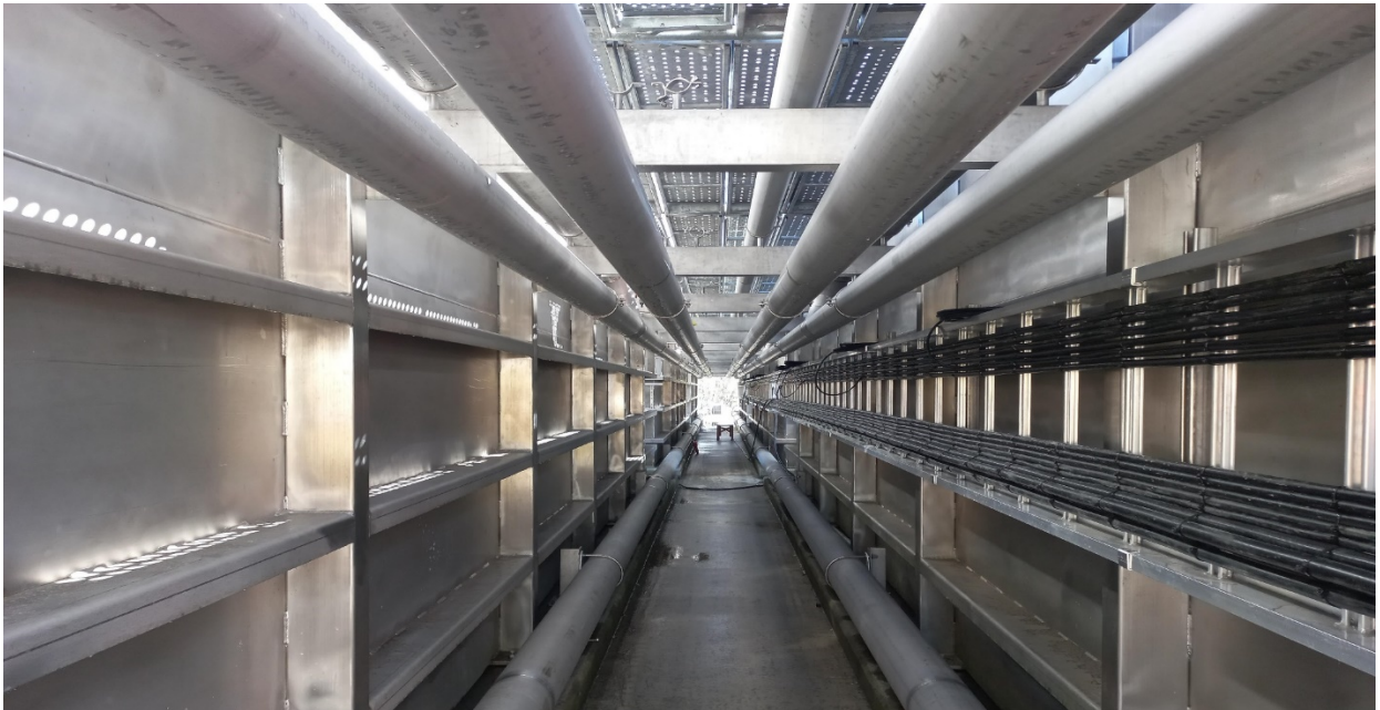
The new MABR tanks service gallery is fitted with process and utility air, power and control lines. Te Kauwhata WWTP
