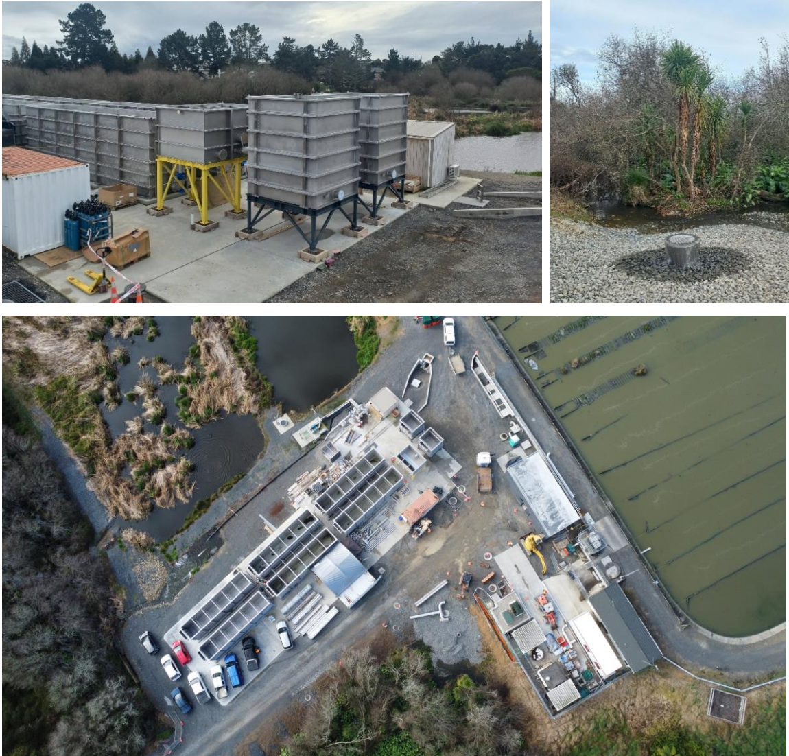
The new MBR tanks and flow splitter tanks, and the discharge pipework were renewed at the Te Kauwhata WWTP
