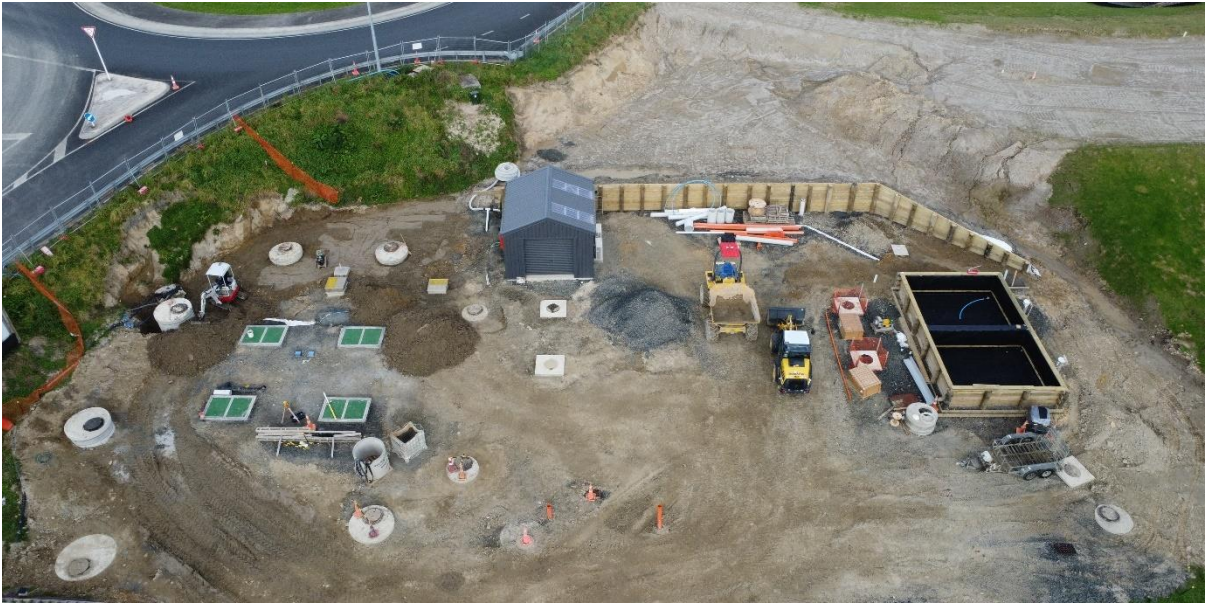
POAL WWPS – The installation of sewers to receive flow from Horotui is underway, along with the new road formation
