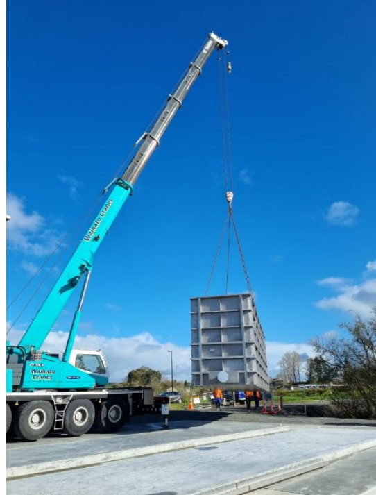
Te Kauwhata WWTP Liquid Stream Aeration Tank
