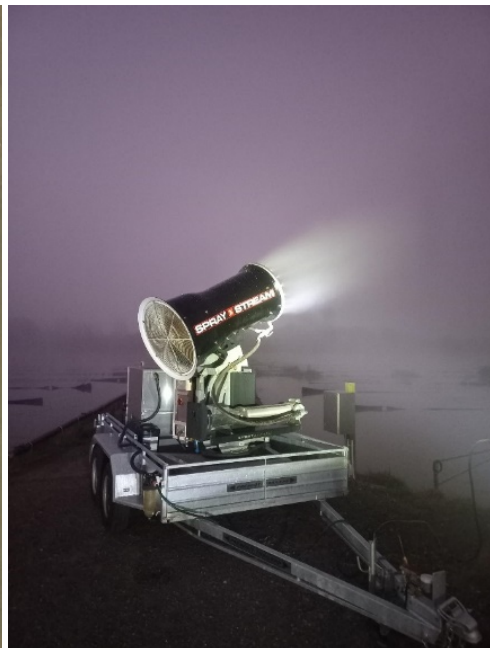
Te Kauwhata WWTP ponds odour cannon
