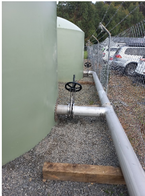
Ngaruawahia WTP – New run-to-waste tanks to store backwash water before a steady release to the local sewer.
