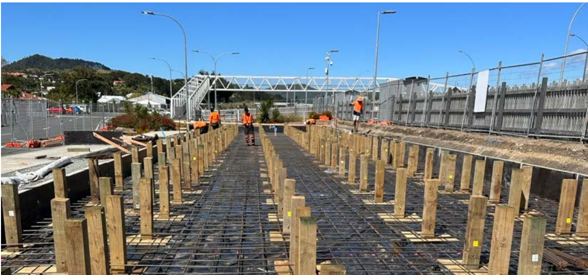
Timber piles and steel reinforcing in place ready for concrete pour on Monday 20 March
