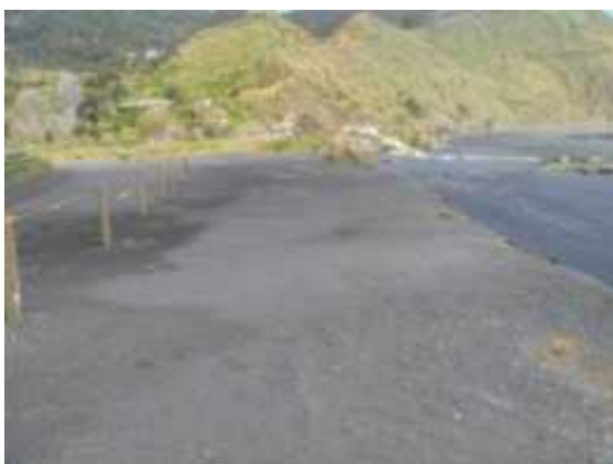
Photograph 6: Failing car park edge looking south (low tide). No pedestrian access to the beach available from this car park now.
