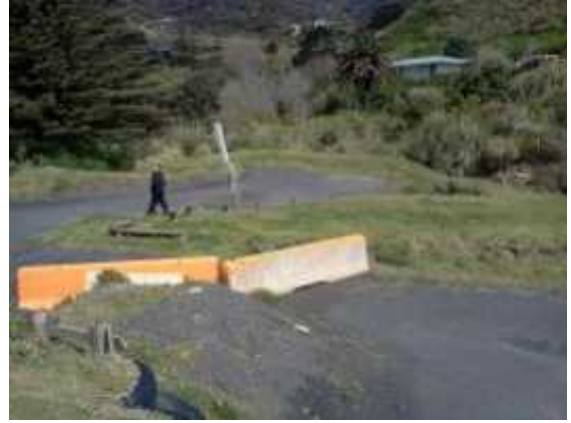
Photograph 9: Sand being deposited against temporary concrete barriers in the middle of the upper and lower car park, southern end. Looking towards the beach access.
