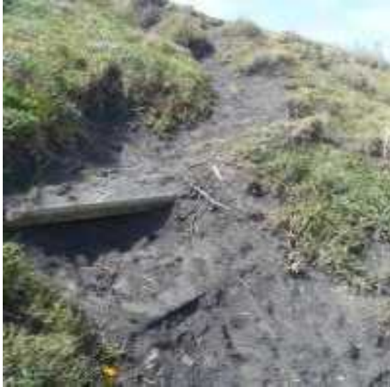
Photograph 14: Concrete telephone poles showing through eroded areas of sand dune below the car park
