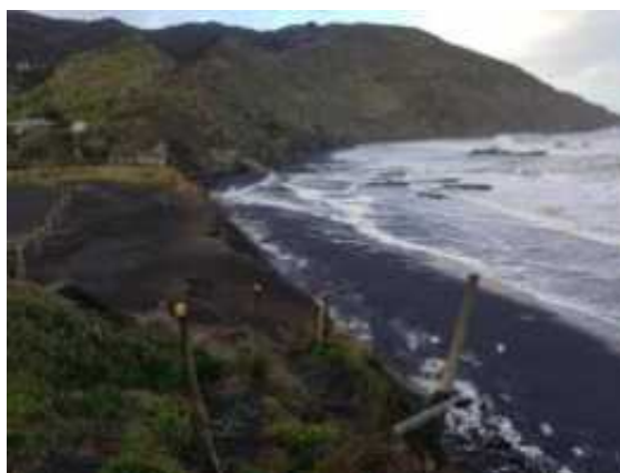
Photograph 7: Failing car park edge looking south (high tide). No pedestrian access to the beach available from this car park now.
