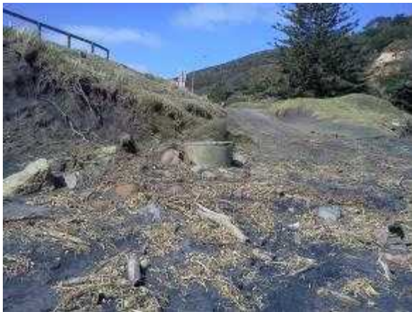
Photograph 12: Site visit in 2014 showing stormwater culvert being covered by further sand.
