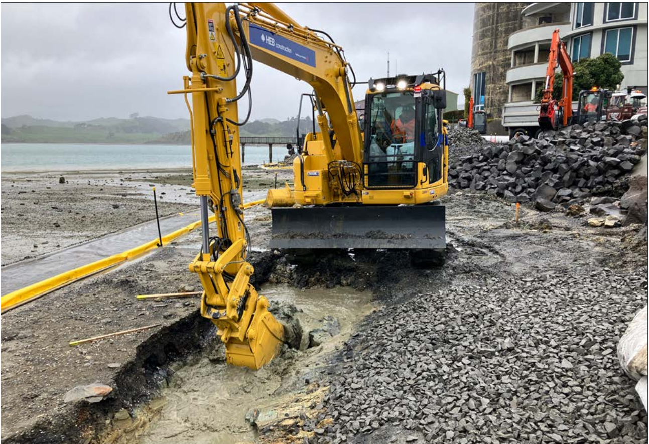
Excavation to the papa shelf to create a hold for the toe boulders.
