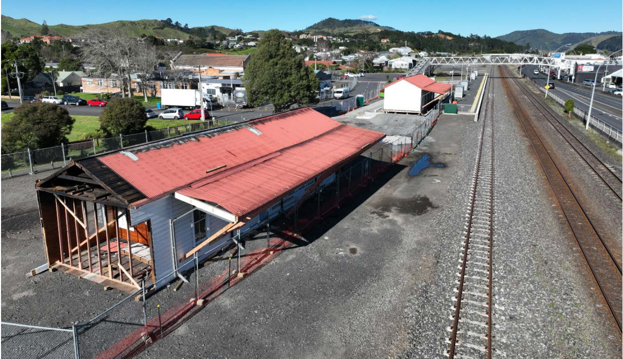
Fire damaged section awaiting insurance assessor.
