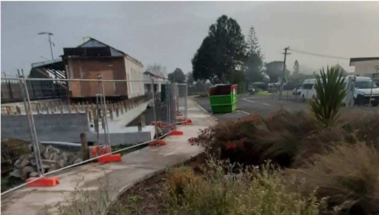
End of second section of the building has been temporarily closed in.
