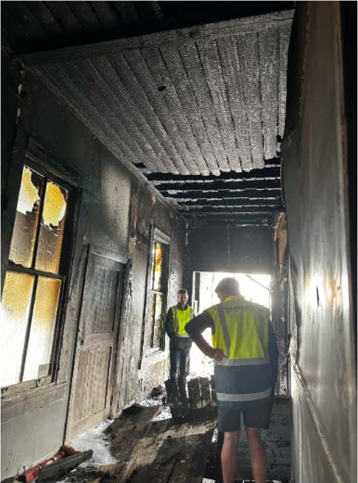
Interior damage from the fire
