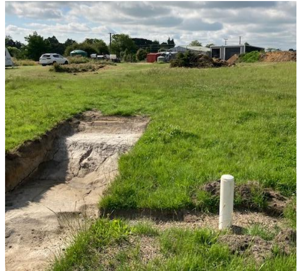
From bore to Implement shed and first filtration system, then to tank supplying house & club house.
