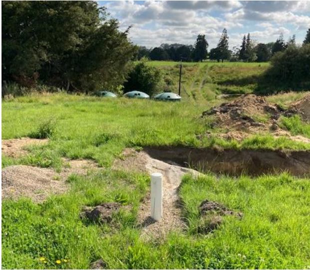
From bore to storage tanks.
