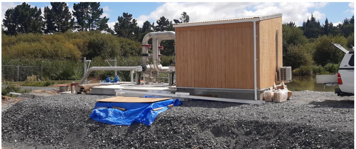
Te Kauwhata WWTP – New UV Treatment System
