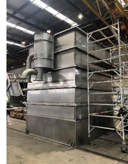
New BAC Filter
