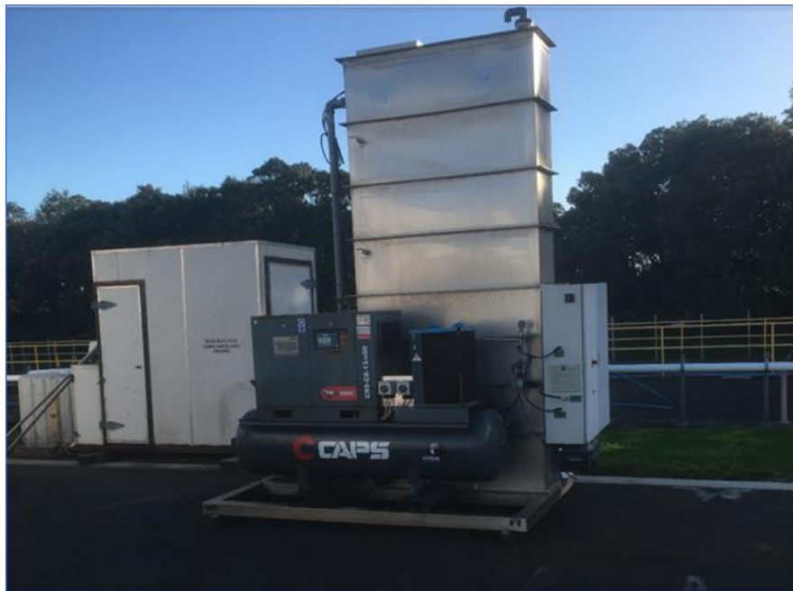
MABR Module in situ at the Innovation centre
