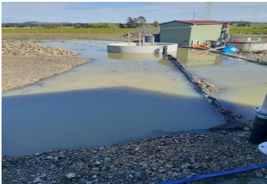
Meremere Wet Land construction site flooding 24/09/2021
