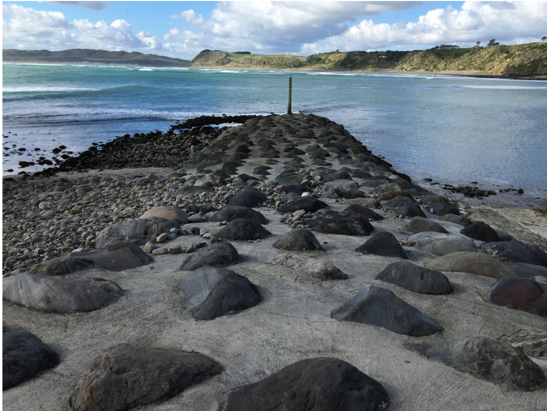
Figure 9: Photo showing the migration of rock material over the upper portion of the breakwater.
