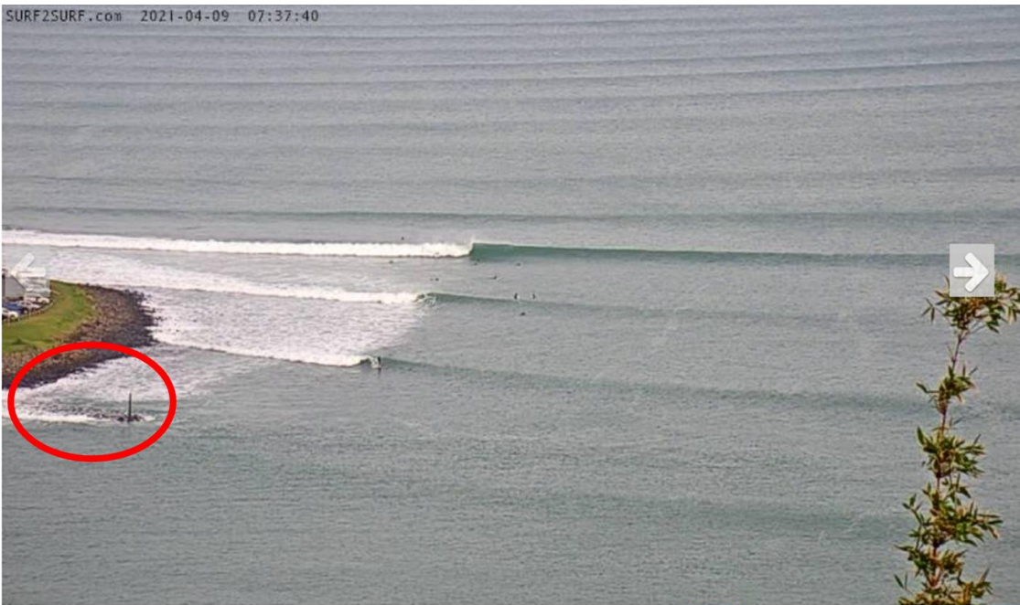
Figure 3: Overtopping of the breakwater structure 1hr before a neap high tide during moderate swell conditions observed on 9/04/21.
