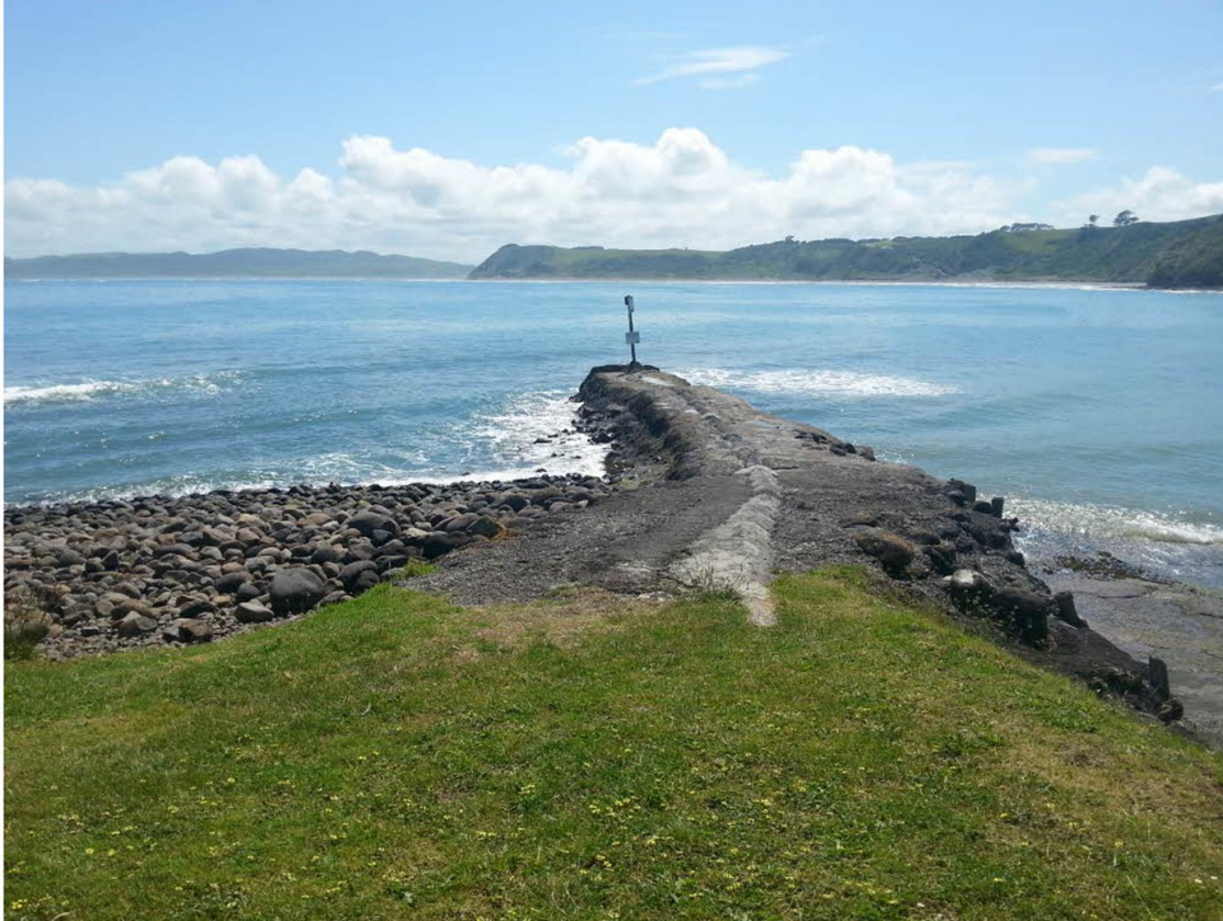
Figure 11: Photo showing accumulated rock material at the western base of the breakwater prior to reconstruction. (Source: WDC).
