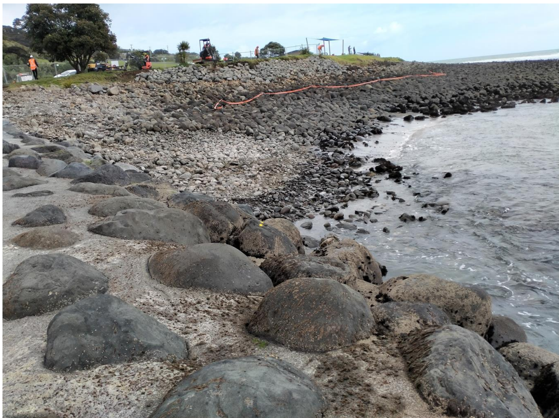
Figure 10: Exposed smaller rock from below the area of excavated larger rock. Note the protection structure constructed from the excavated rock along the upper the bank in the centre top portion of the image.
