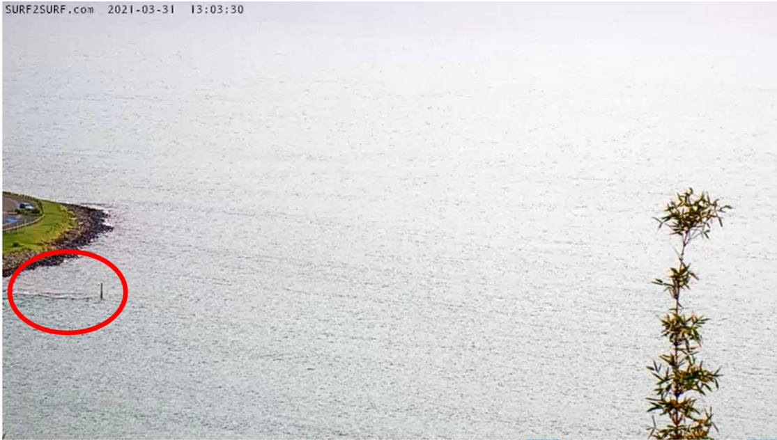
Figure 2: Overtopping of the breakwater observed on 31/03/21 during minor swell and spring tide conditions.
