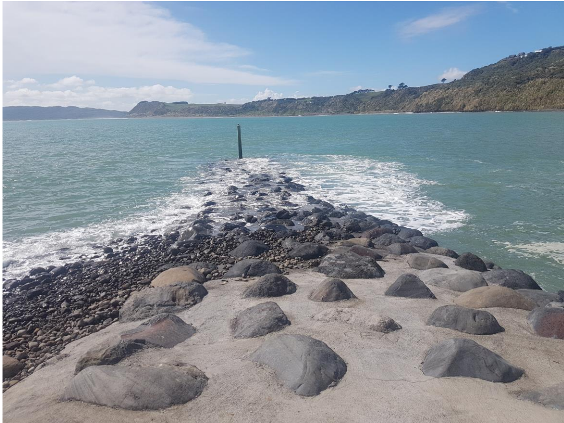
Figure 8: Wave overtopping event at the Manu Bay breakwater. Note the extent the white water line on the inside of the ramp indicating the dissipation of broken wave energy as the wave moves over the breakwater and into deeper water. The extent of wave penetration past the breakwater will be highly dependent upon swell conditions at the time.
