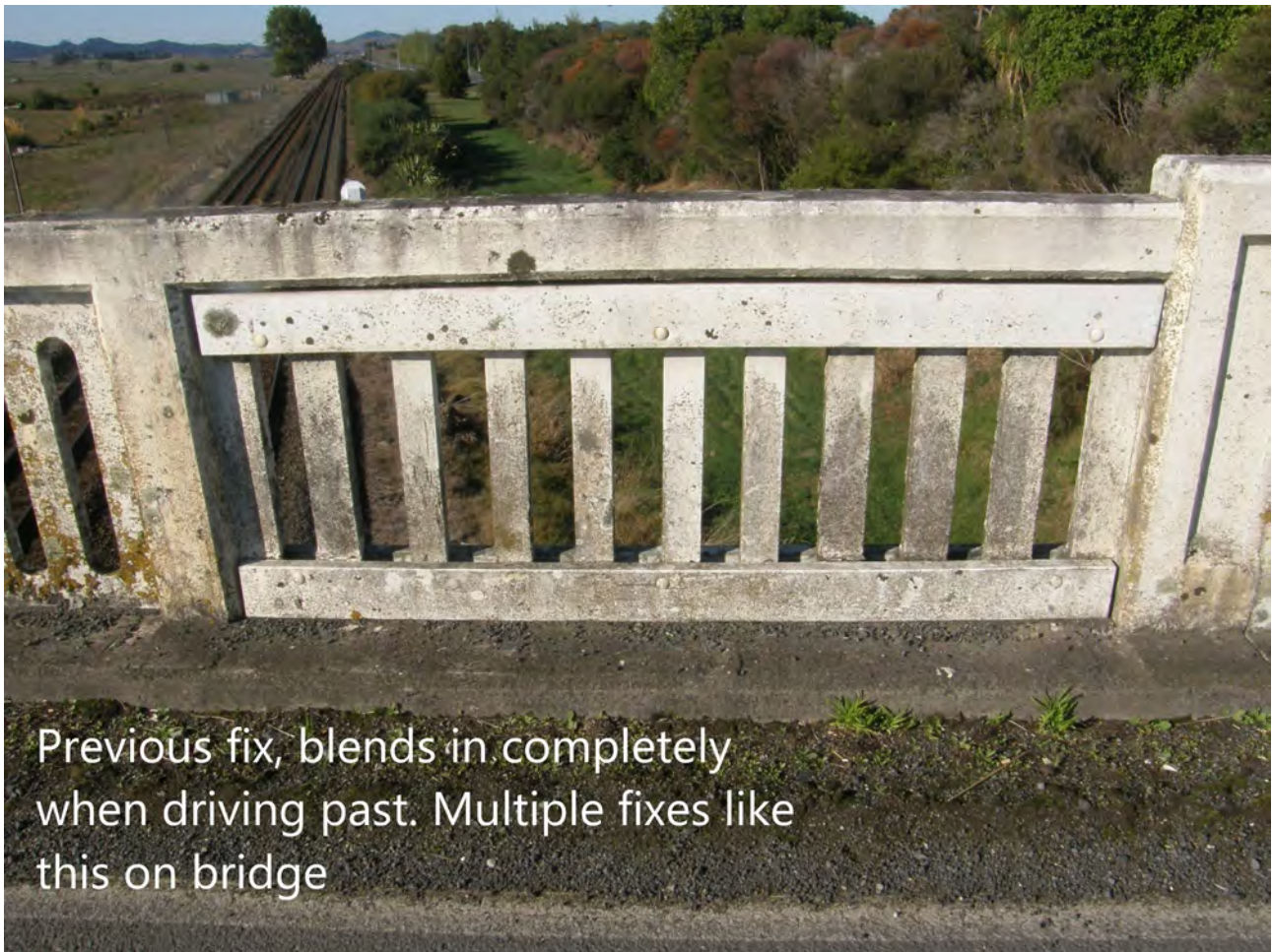
Example of another fix on the bridge to the same problem (photo sent to council)
