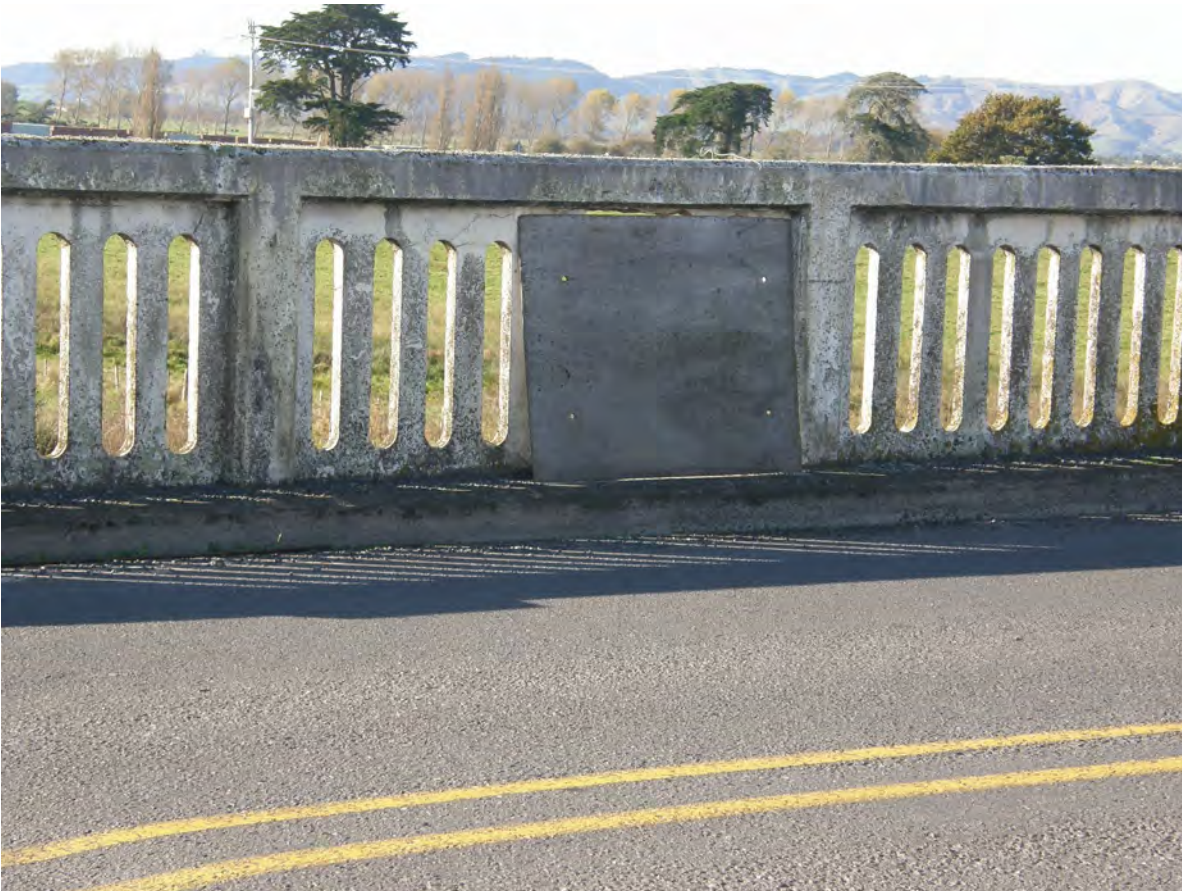
Current state of hole in Ohinewai bridge
