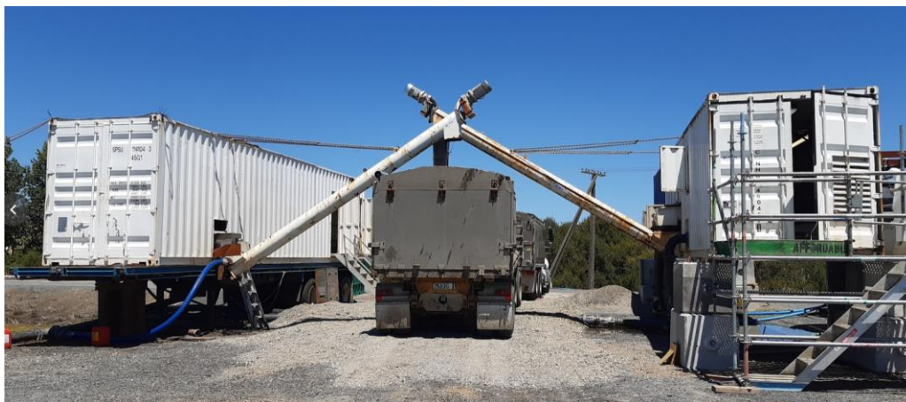
Huntly WWTP – Centrifuge Sludge Processing
