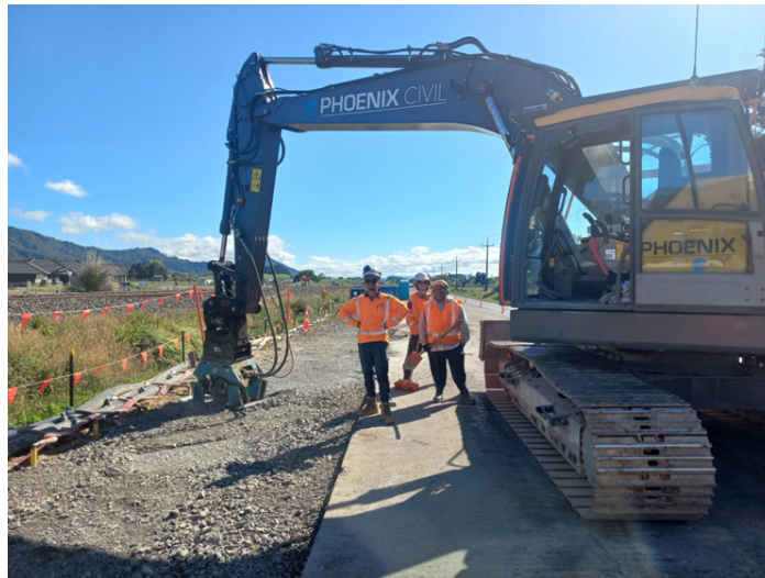
Ngaaruawaahia Pipeline – The installation works under a Great South Road Lane closure.
